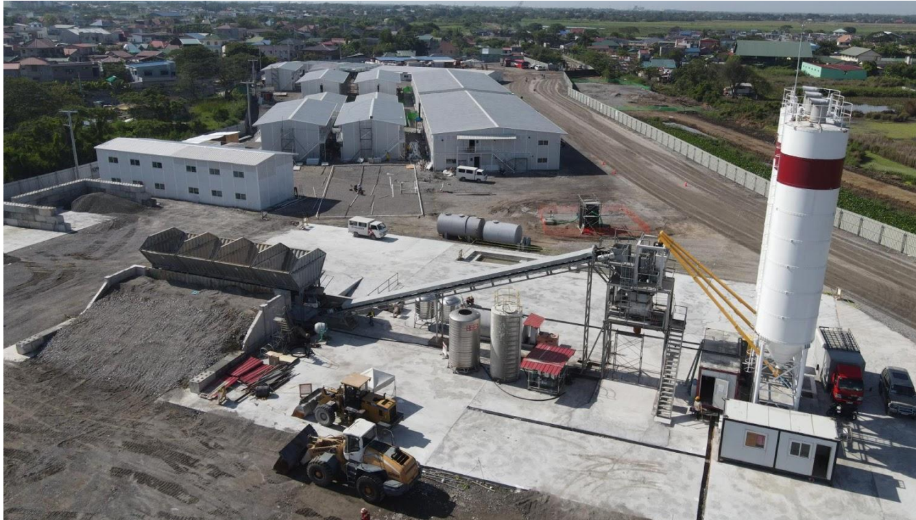
CPN01 Batching Plant
